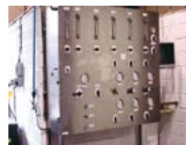
High Pressure Gas Test Panel capable of 500 barg (7150 PSI) with video link to Test Cell
